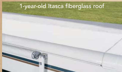
1-year-old Itasca fiberglass roof
