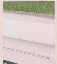
One-year-old Winnebago Industries fiberglass roof
